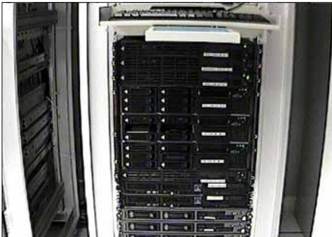
Optic image of a network hard drive rack.
